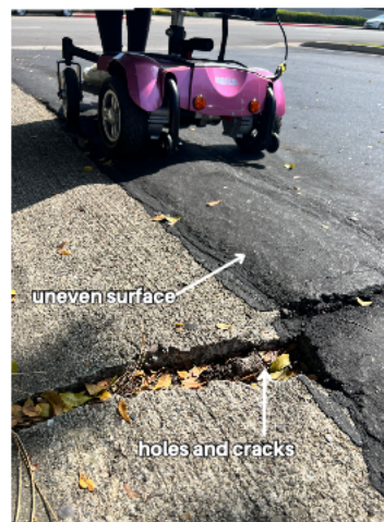
Figure 2. This image shows holes, cracks, and an uneven surface along a parking lot. Users must be aware of their PWC tilting on these types of uneven surfaces.
